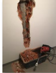
Sewer pipes within the buildings
